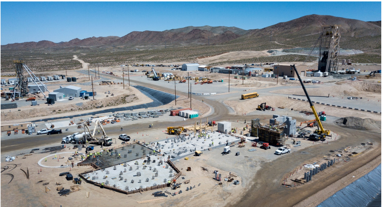
(East North and Main Shafts shown in background. Process Plant in foreground)
